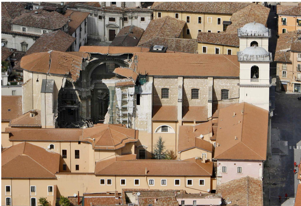
Figure 1. The Duomo Cathedral of San Massimo is seen damaged in the town center of L'Aquila, central Italy, on Tuesday, April 7, 2009. (AP Photo/Alessandra Tarantino)
